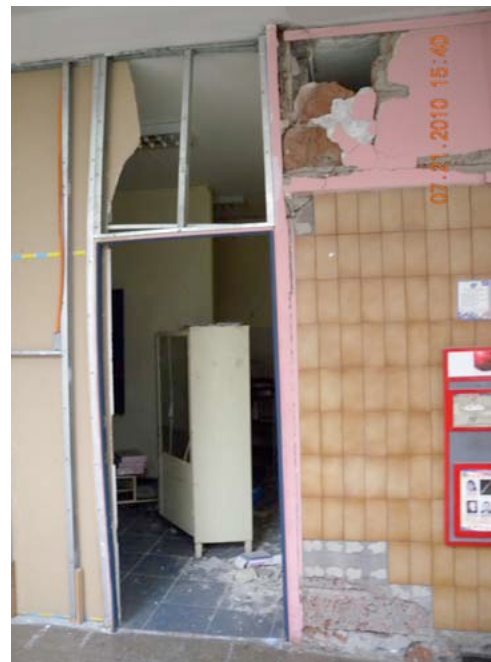
Figure 15. Damage at Felix Bulnes Hospital, outside of Santaigo. As of July 2010, the hospital was still partially closed due to unrepaired damages.
