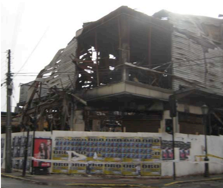
Figure 13. A supermarket in Concepción, which was destroyed in a fire set by looters.
